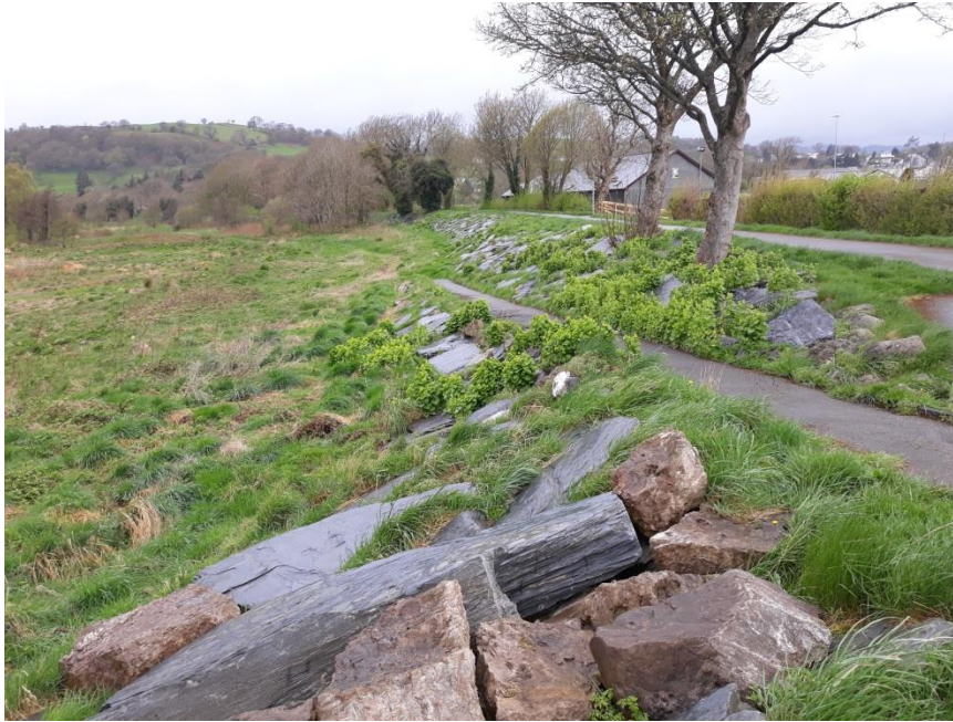
Plate 3.3: View of embankment upstream face where ramp provides access to crest (close to ‘bandstand’); slate rip-rap has been supplemented with imported granite
