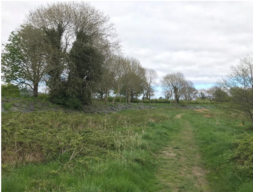
Plate 3.1: View from the foreshore looking east along the lake embankment upstream face
